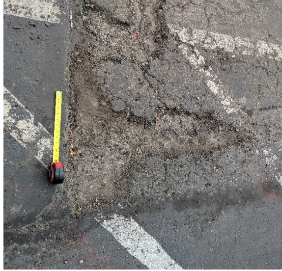
Figure 2.8 Scanned pothole with a tape measure providing one foot as a reference
