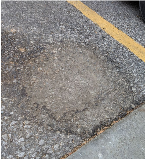
Figure 2.10 The second scanned pothole
